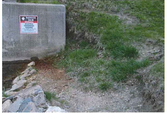
April 27, 2015 Shore erosion adjacent to abutment.
