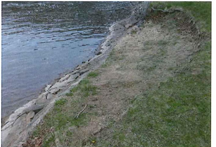
April 27, 2015 Shore erosion above the grouted rip rap
