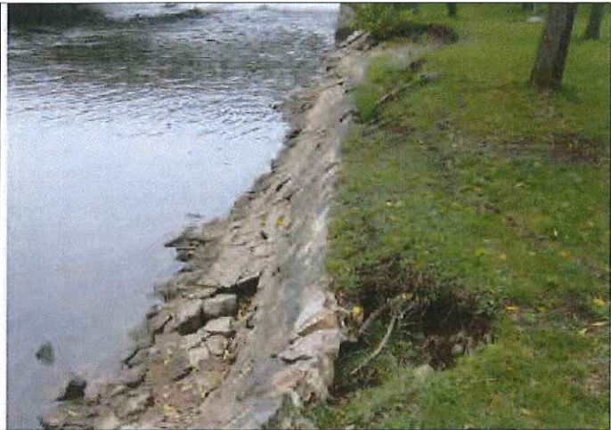
August 27, 2013 Damage to grouted rip rap
