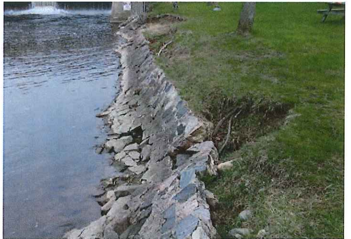
April 27, 2015 Damage to grouted rip rap
