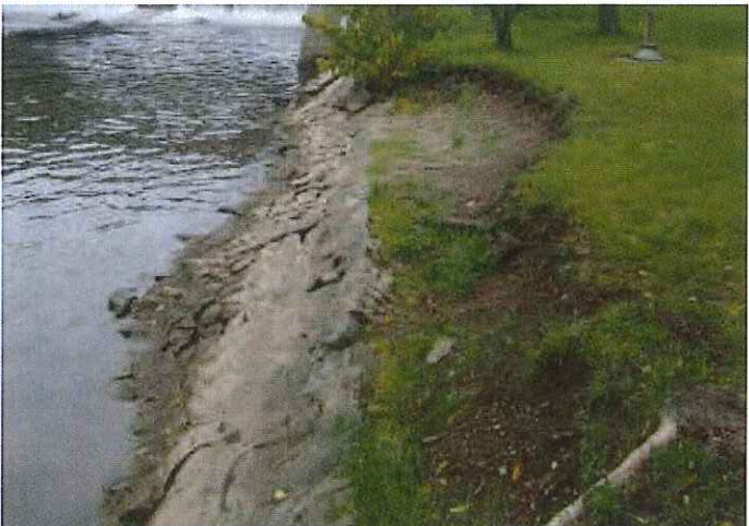
August 27, 2013 Shore erosion above rip rap
