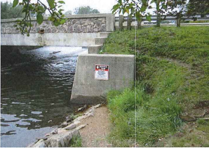
August 27, 2013 Shore erosion adjacent to abutment
